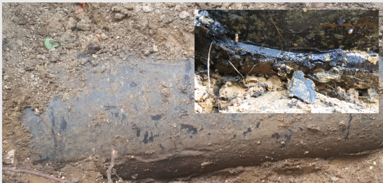
Figure 1: Pipeline Coating showing signs of loss of adhesion (disbondment); Inside picture shows presence of an aqueous environment under disbonded coating where external SCC may initiate
