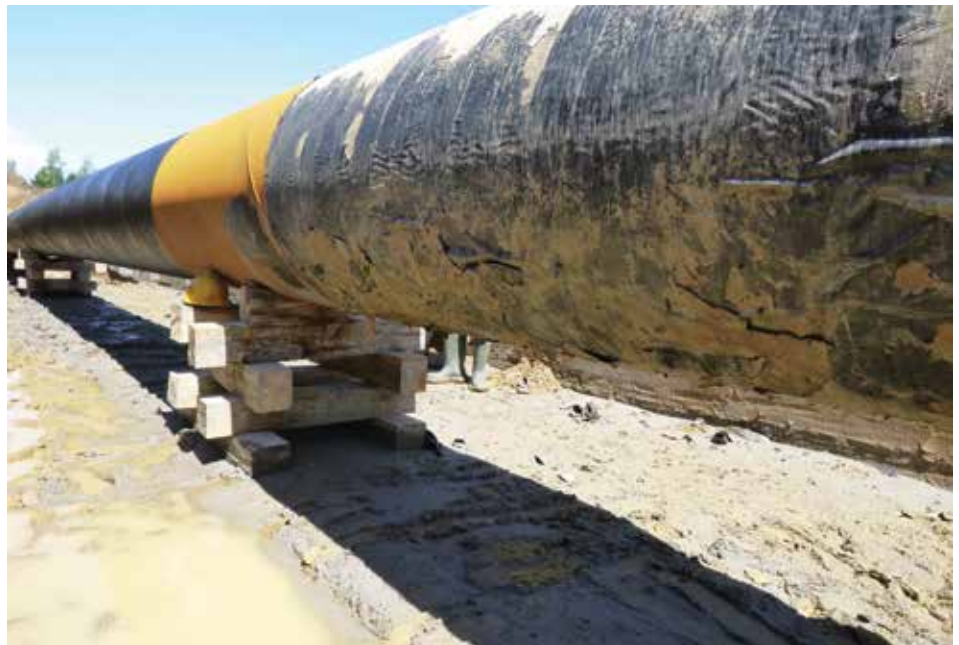
An ageing, deteriorating pipeline.
