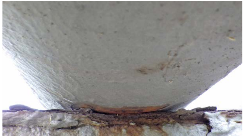
Figure 4. Image of the pipe support with 40% wall thickness loss from the exterior.
