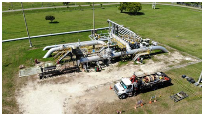
Figure 1. Loading lines only have one launch/receive site, making bidirectional inspection necessary.
