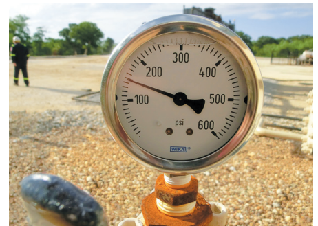
A gas pipeline operating at pressures lower than normal often does not allow for a traditional ILI.
